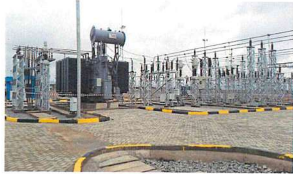
The power sub-station at the Naivasha SEZ
