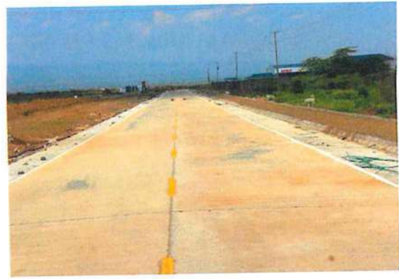
Completed and marked road section of the Access Road 2 leading to Jumbo AAA SEZ Ltd
